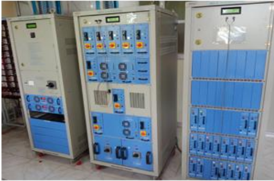
INTEGRATED POWER SUPPLY PANEL
