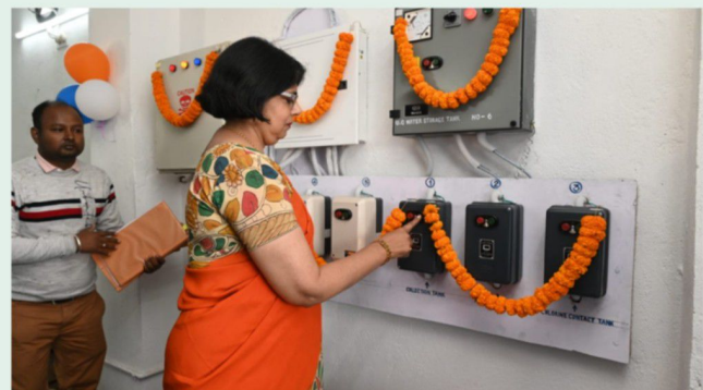
Ms. Archana Joshi, General Manager, South Eastern Railway inaugurating the Water Recycling Plant at Bankura on 06.01.2023.
