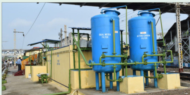
Water Recycling-cum-Effluent Treatment Plant at Santragachi
